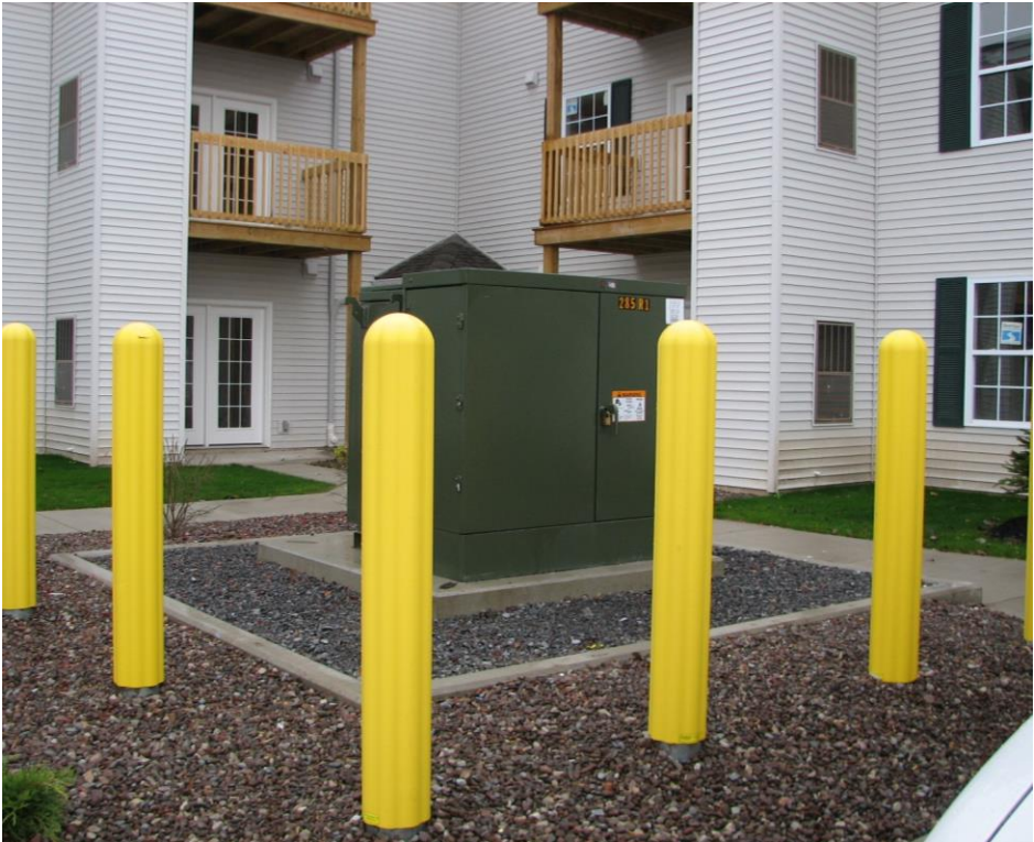
Picture of Ballard Installation
